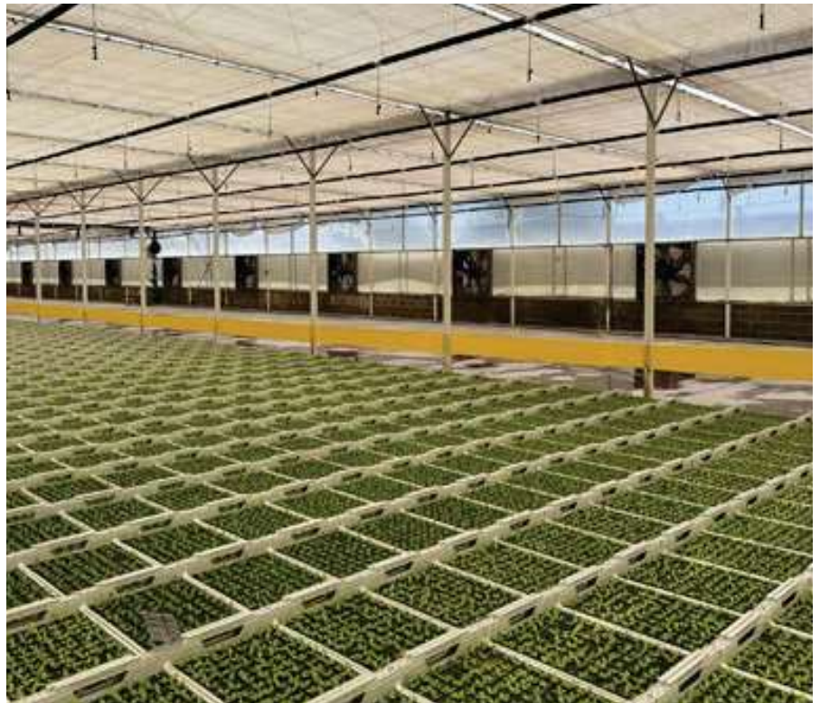
To minimize problems with too high temperatures in the summer the nursery has a pad & fan system.
